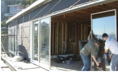
Two Old Town Glass technicians install a sliding glass door on a client's home.
