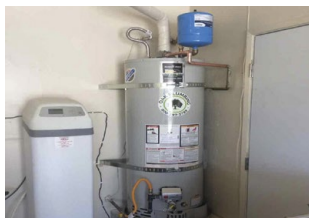
Oak Plumbing installed this water heater in a customer's garage.
