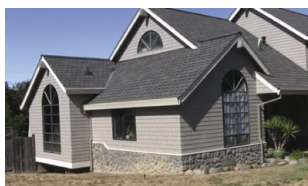
ABS Home Pro installed this contemporary seamless gutter system to enhance beauty and manage rain flow.
